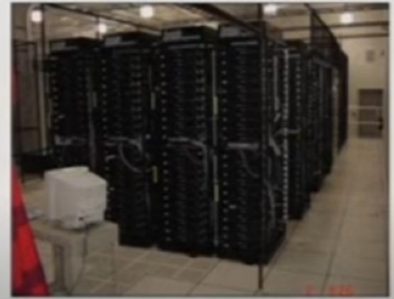
Google data Center (2008)
